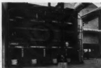
B&W air heater heats combustion air for copper anode furnace and cools flue gas for zinc oxide recovery.
